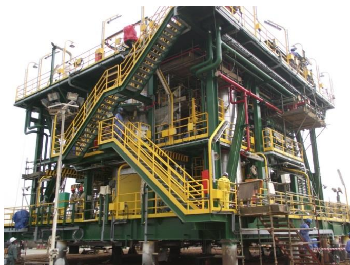
Figure 6 – H 2 S Removal Module
