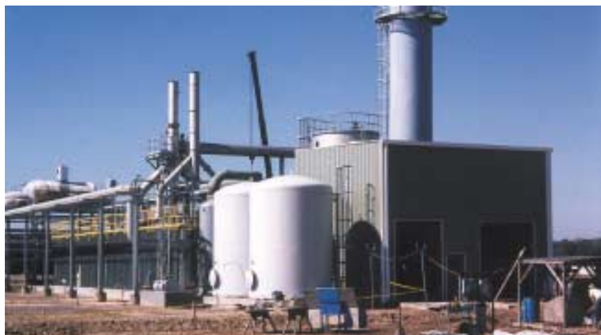
The first LO-CAT unit to treat Claus tail gas was recently installed at the Western Gas/Anadorko Bethel plant in Texas, USA.
